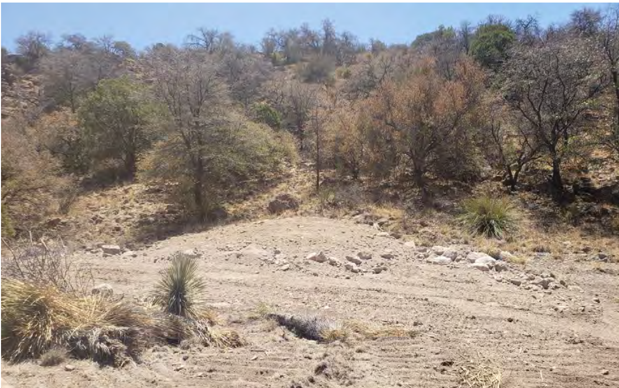
Photo 2: Crew mounded cover material in areas where former mine workings potentially persist.
