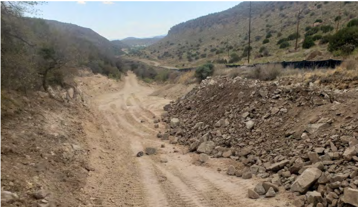
Photo 2: With new grading plan at north end of site, the road (right) will ramp in along east bank and creek will flow along former road (left).
