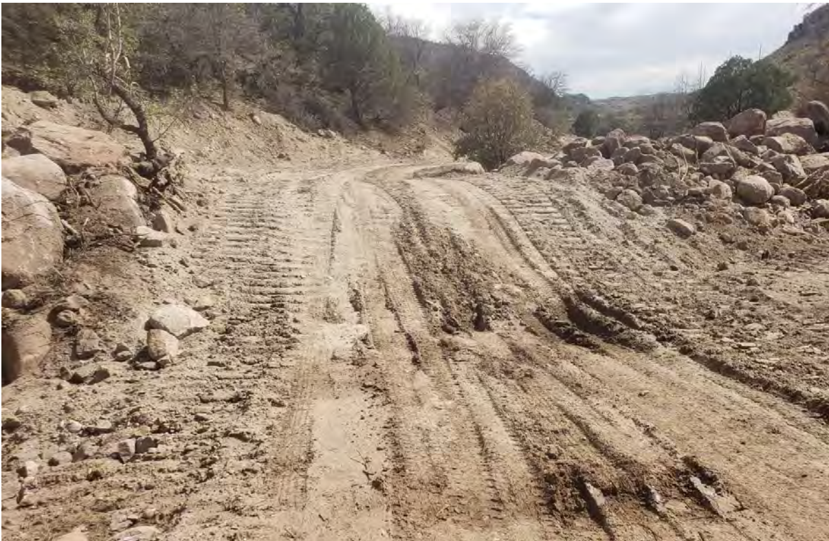
Photo 4: A new berm on the access road will enable seeding crew entry and keep creek in channel.
