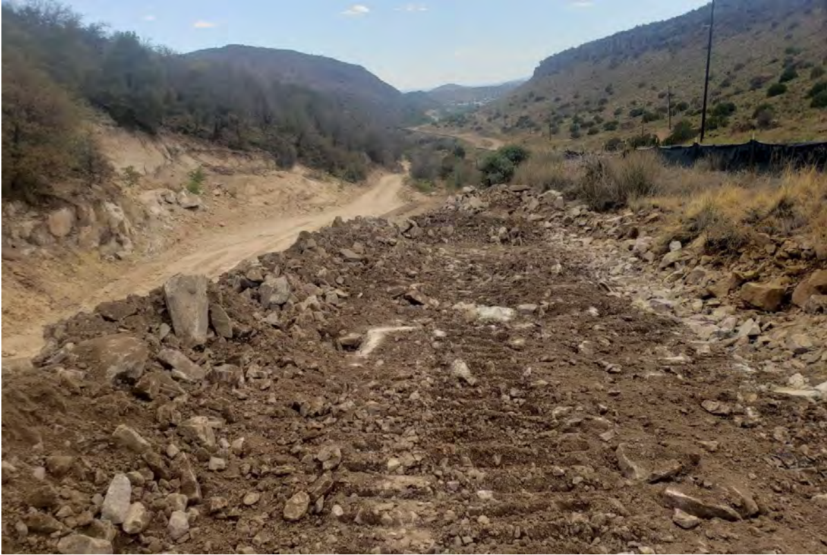
Photo 1: Shared Services hauled 53 loads of cover material to ramp at north end into site.
