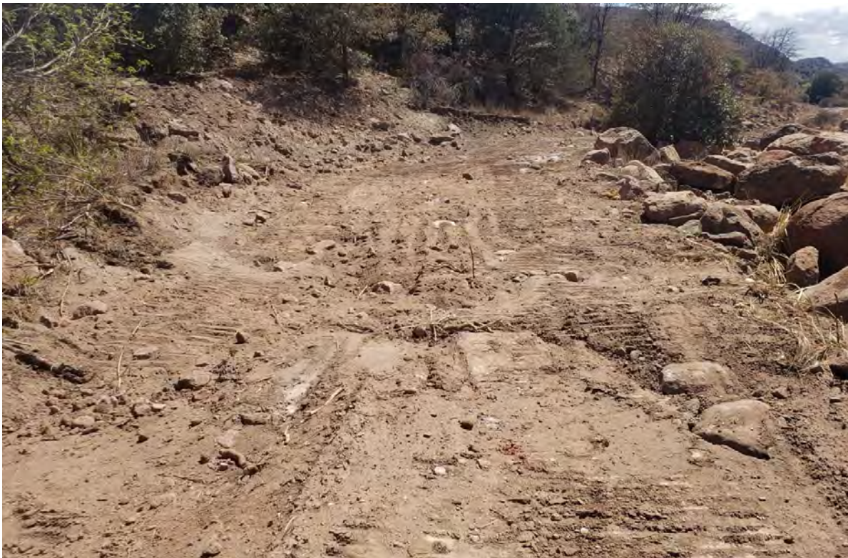
Photo 4: Shared Services rebuilt the access road after removing ~2 feet of reddish material.
