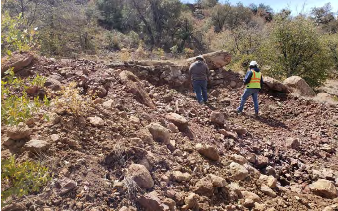
Photo 1: David Mercer (NMED) and Travis Wilmes (Shared Services) inspected concrete foundation at Shaft 2 where partial removal was completed previous day.
