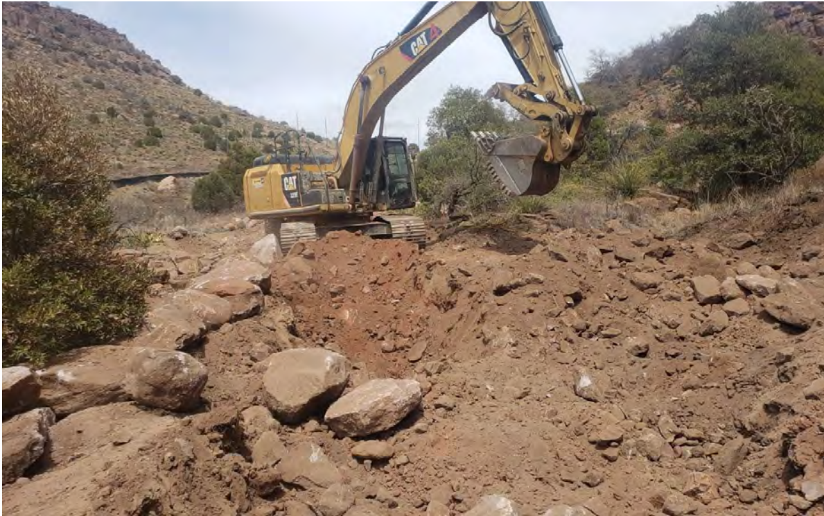
Photo 3: While removing surface material from small flagged locations along access road, Shared Services encountered unexpectedly thick layers of reddish material.
