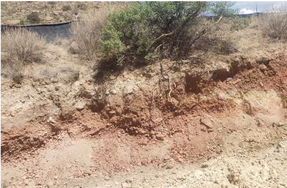
Photo 2: Wall adjacent to pipeline corridor where reddish material (native and stockpiled) remains will be capped with clean, import material.
