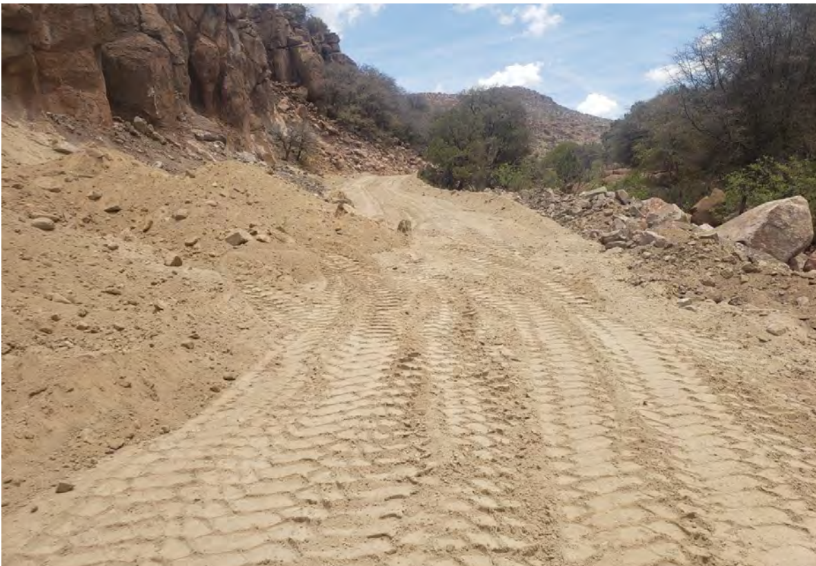
Photo 2: Crew added mounds of material (left) along former workings going into Lucky Bill.
