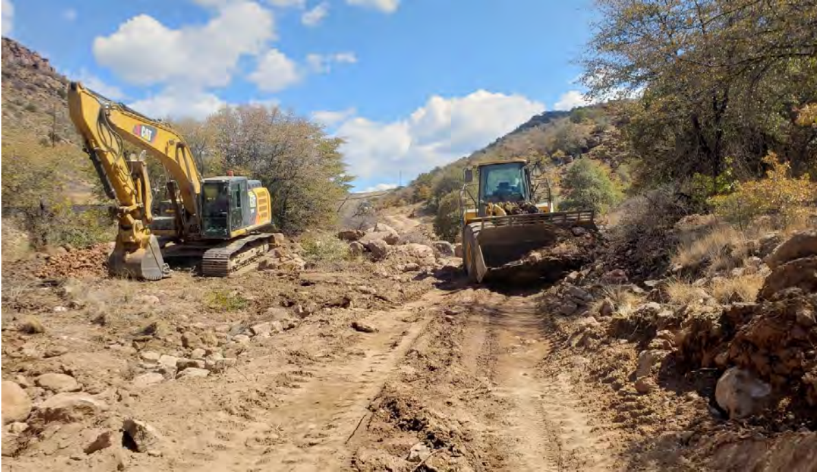
Photo 1: Shared Services removed stockpiled material east of access road (left) while also removing material from around Shafts 4 and 5 on west side of access road (right).
