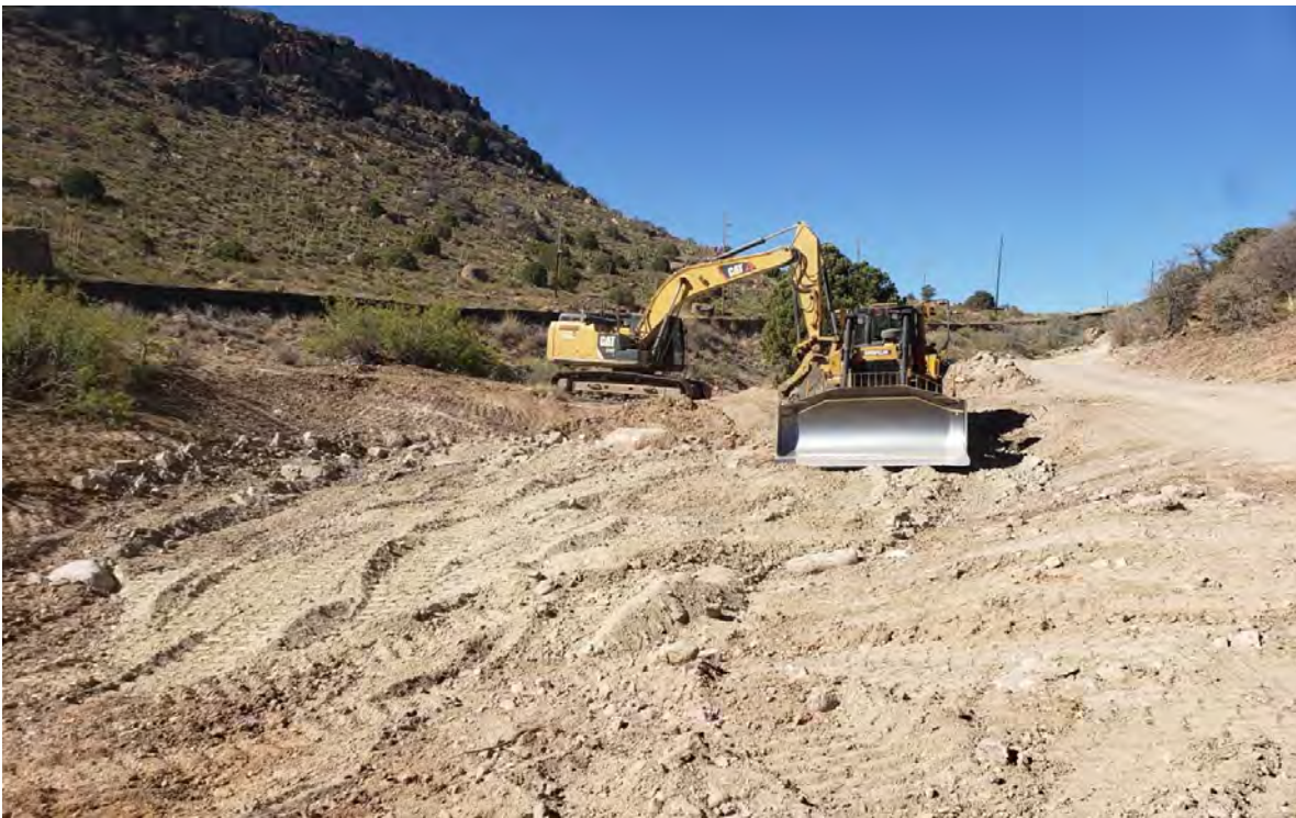
Photo 2: Crew nearly finished filling hole from deep excavation along creek above Lucky Bill.
