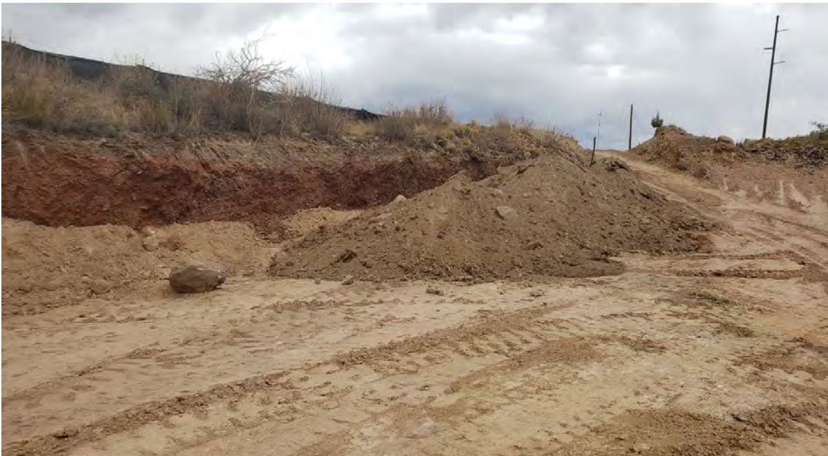
Photo 4: Substantial progress was made backfilling along red wall at north end of jobsite.
