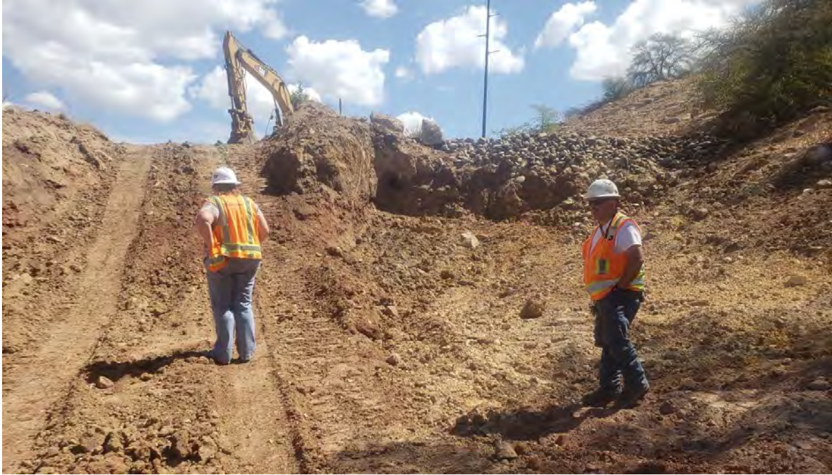
Photo 1: Chino, Shared Services, and DBS&A walked northern half of work area and compiled final punch-list for excavation activities.
