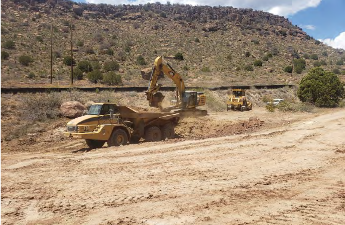
Photo 1: Shared Services began removing 8'-thick layer of yellowish material from platform in creek bed near entrance to Lucky Bill Canyon.
