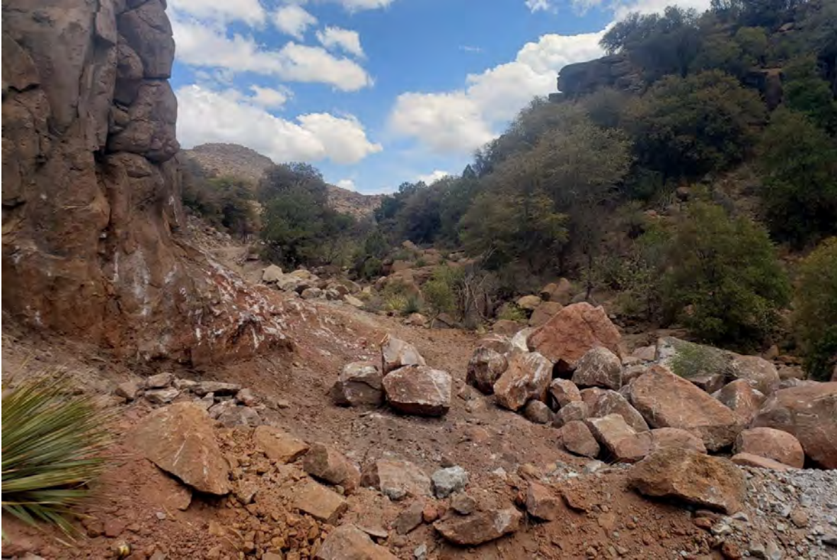
Photo 1: Shared Services continued removing material from the former road near Shaft 3 at the confluence with Lucky Bill Canyon.
