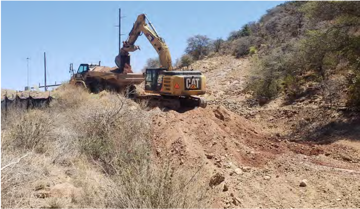
Photo 1: Over past 3 work days, Shared Services removed nearly all remaining red material at Shaft 1 east, west, and beneath access road.
