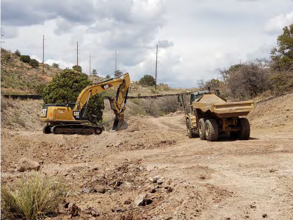
Photo 3: After completion of excavation at north end of jobsite, Shared Service returned to Lucky Bill confluence and removed reddish material from numerous small areas flagged for punch-list.
