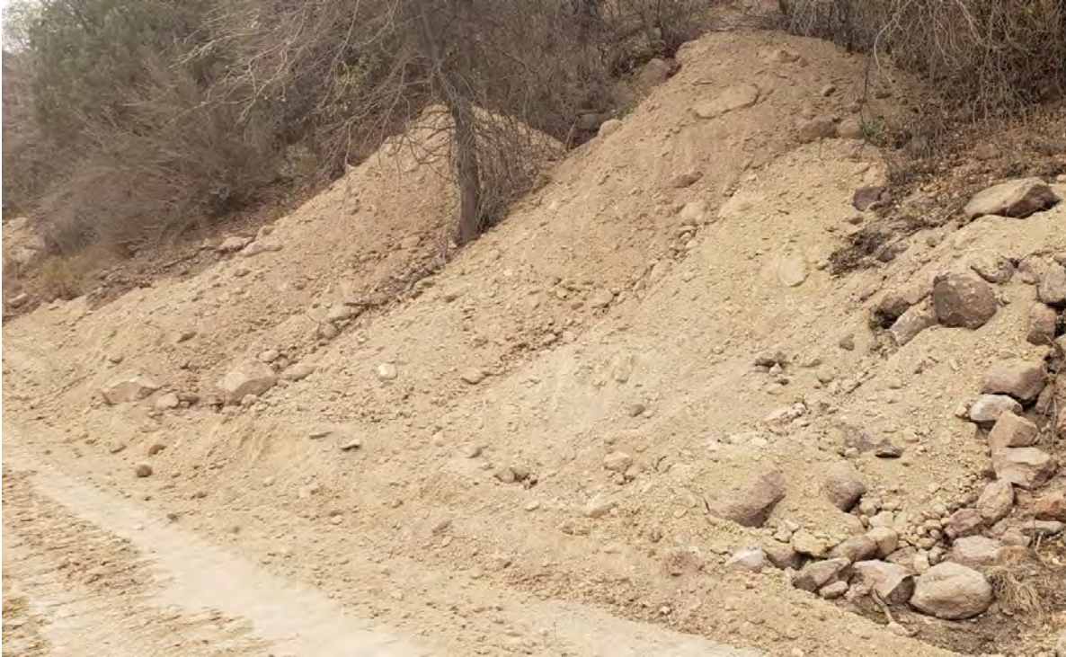
Photo 1: Shared Services placed cover material with mounds over former workings along access road below Lucky Bill.
