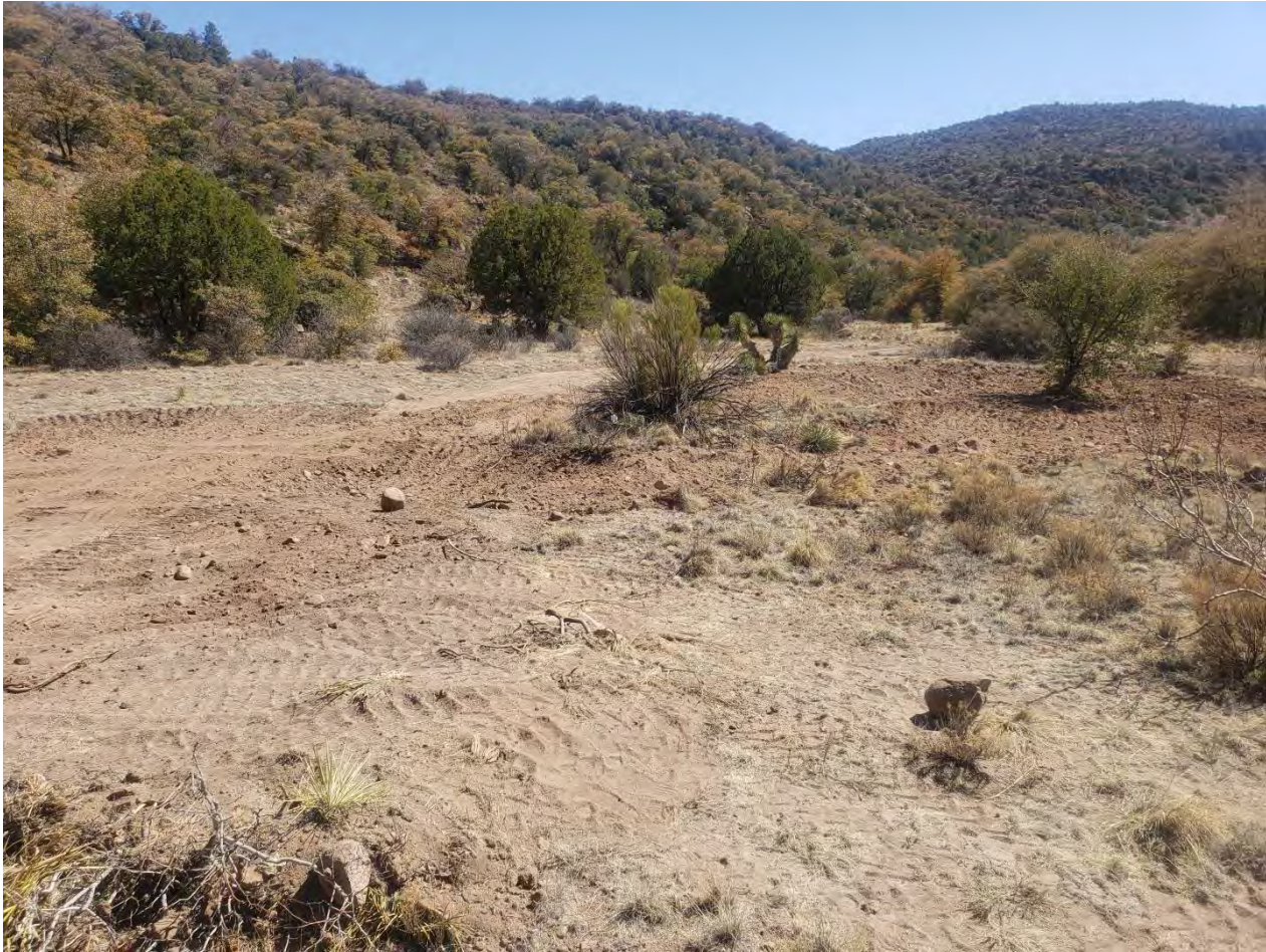
Photo 1: Shared Services removed red material from varying depths across broad area in central portion of jobsite.
