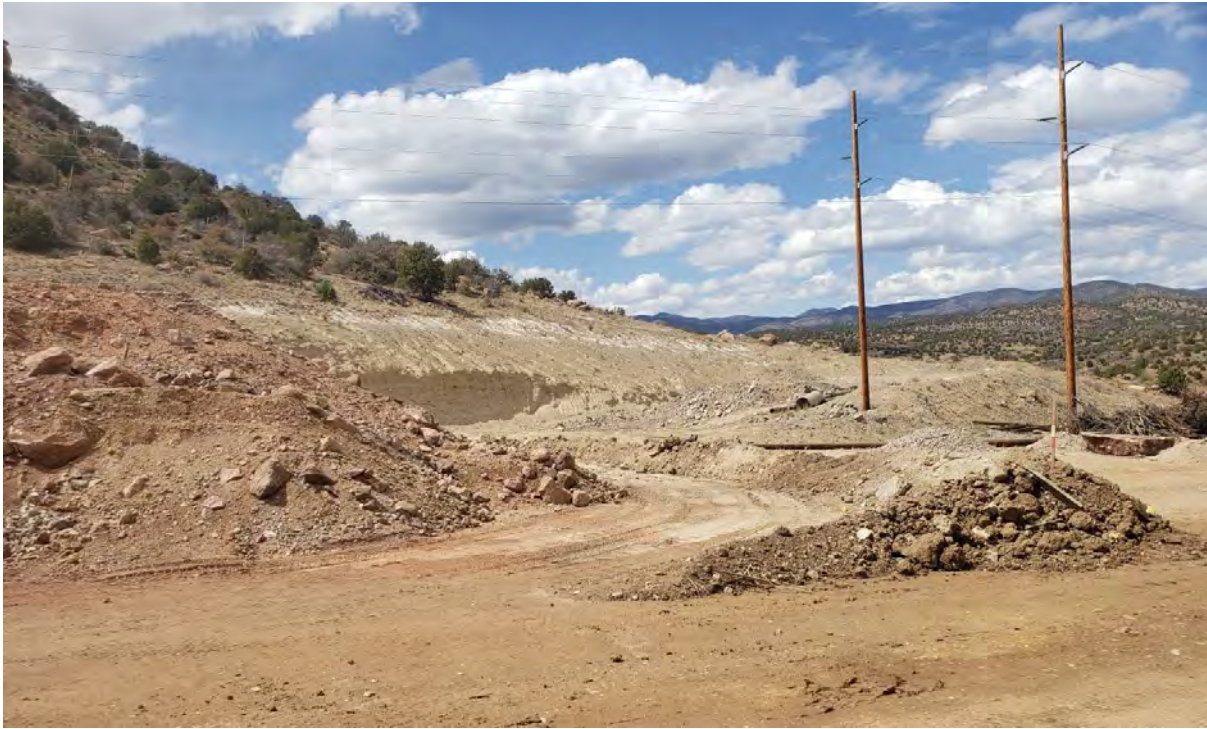
Photo 3: Shared Services built an outer berm (right) for better containment of the original stockpile.
