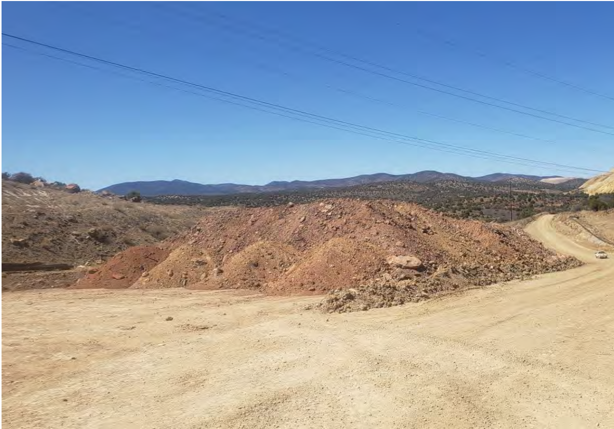
Photo 3: Second stockpile boundary will need to be expanded in the next day or 2 to accommodate additional removal material.
