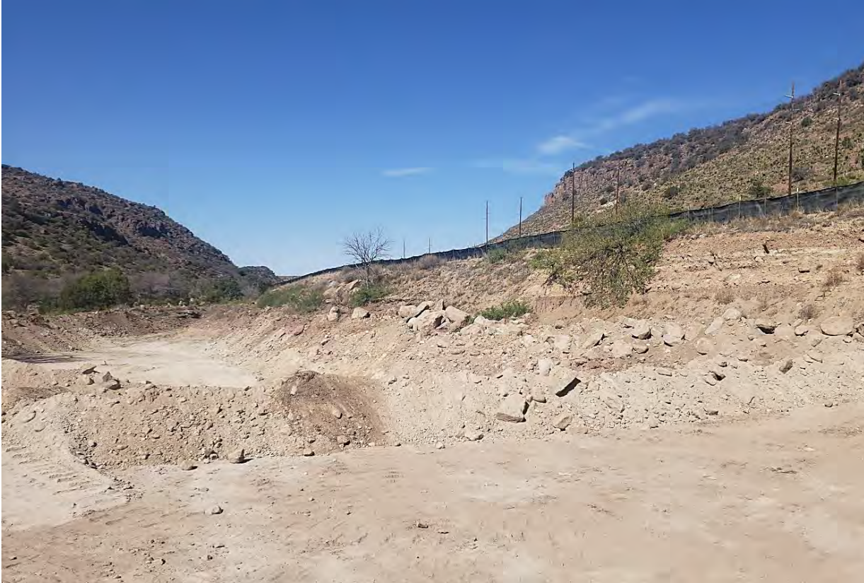
Photo 3: A stout berm along edges of the southern borrow area to prevent stormwater entry.
