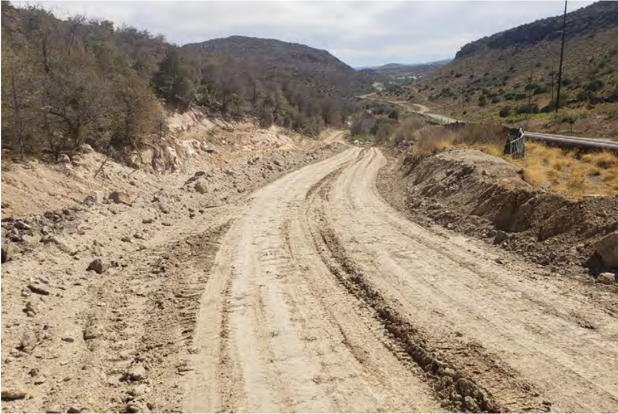
Photo 1: Shared Services finished reconstruction of ramp at north end of work area.
