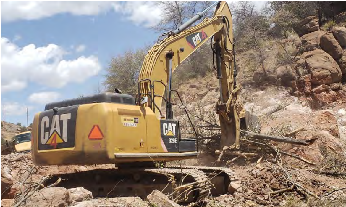
Photo 2: Excavator operator (Miguel) using tree limbs to sweep soil from rocky slope to toe for removal.
