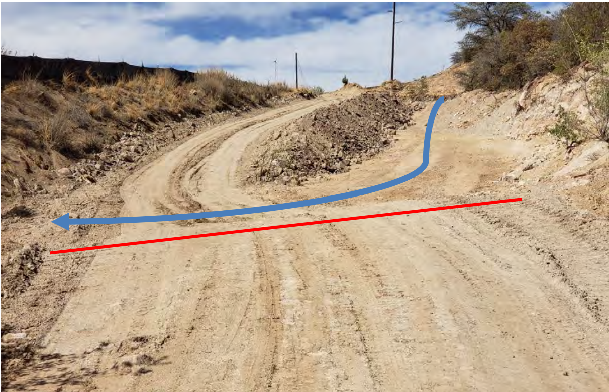
Photo 2: A newly-constructed berm (red line) will help keep creek flow from following access road.
