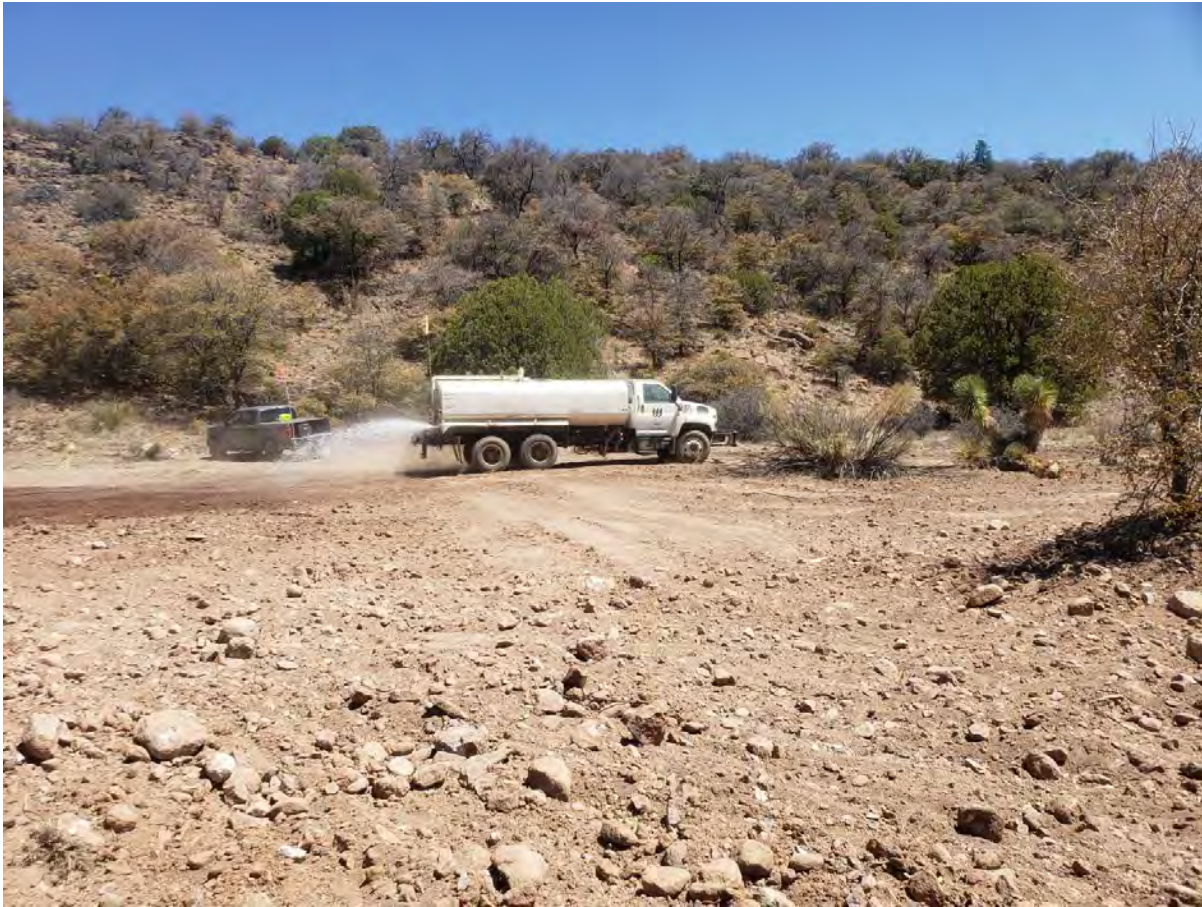
Photo 3: Recently-repaired water truck was used for dust suppression on haul roads and both stockpiles.
