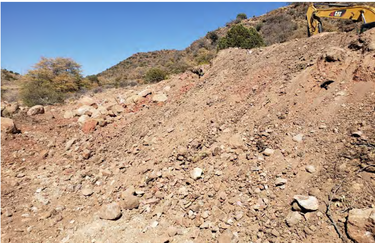
Photo 2: After full day of removing red material from same location along creek bank, red material was beginning to taper off.
