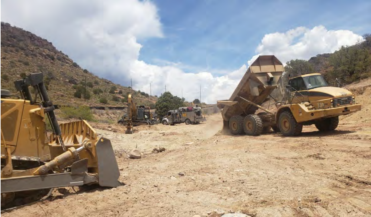
Photo 1: Shared Services finished filling large excavation above Lucky Bill confluence. Mechanics were onsite repairing a/c in excavator.
