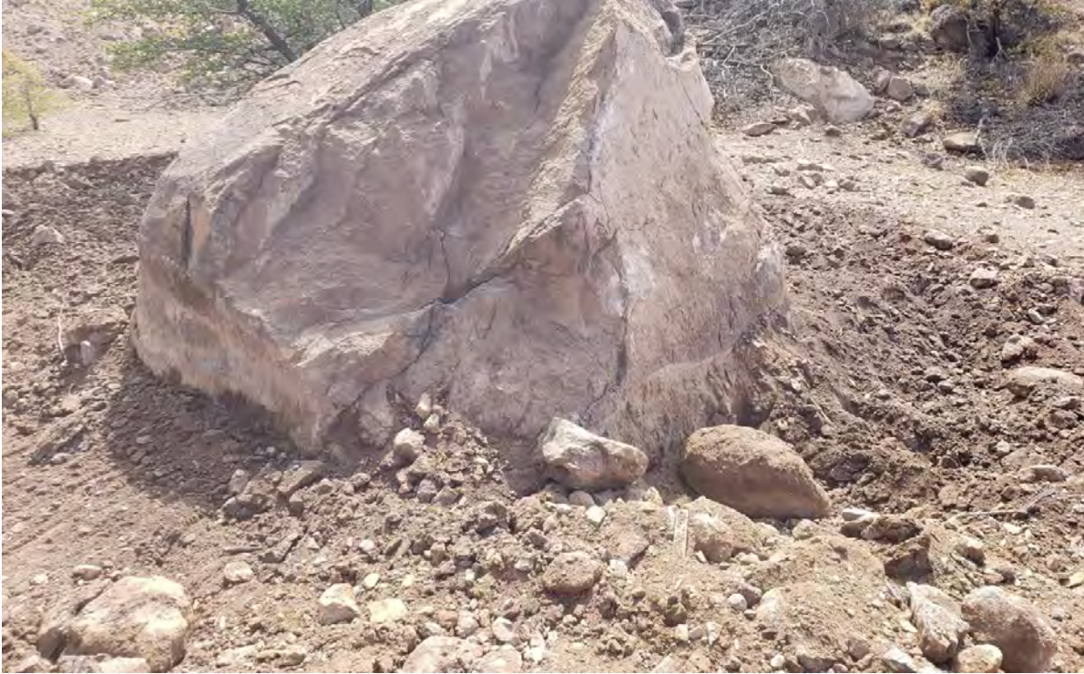
Photo 1: Shared Services removed 1 load of reddish material from the creek bed that had deposited around this large boulder.
