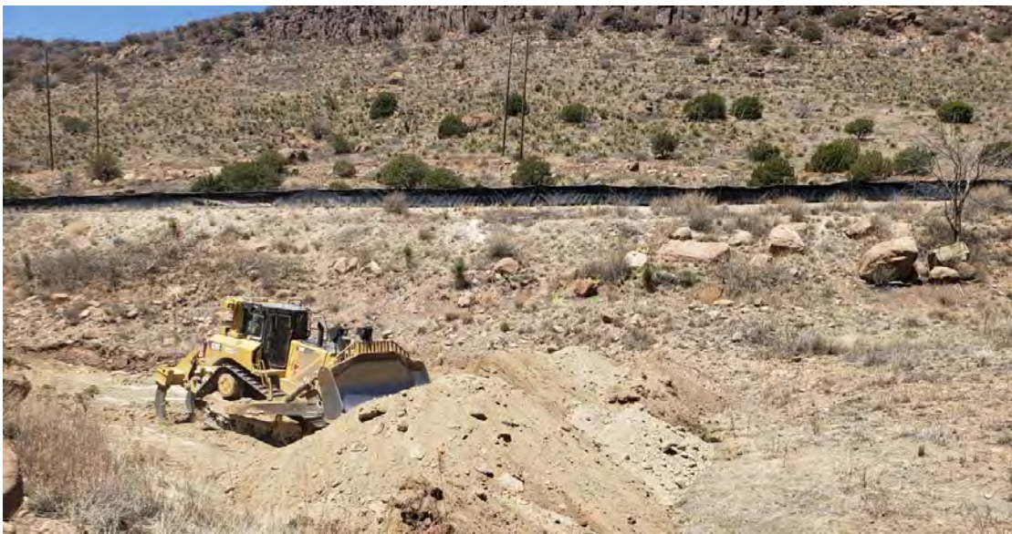
Photo 1: D8 dozer stockpiling backfill material at borrow source as shown in Figure 2.
