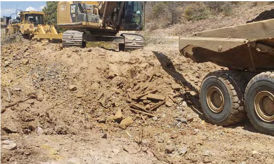
Photo 2: Crew encountered lumber amid yellowish waste material at location shown in Photo 1.
