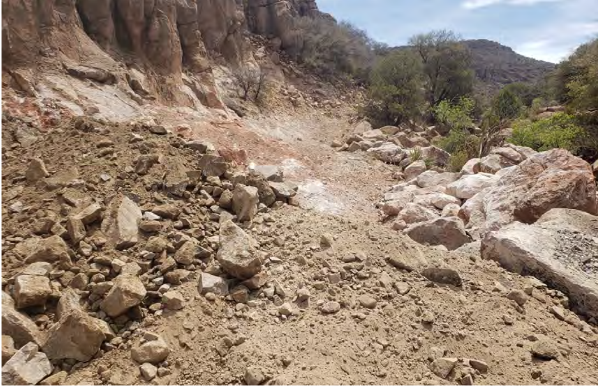
Photo 1: Shared Services spent most of day continuing to rebuild road going into Lucky Bill.
