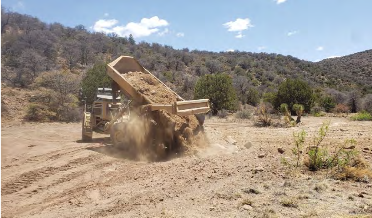
Photo 1: Shared Services hauled backfill material from borrow area to 3 southernmost removal areas.
