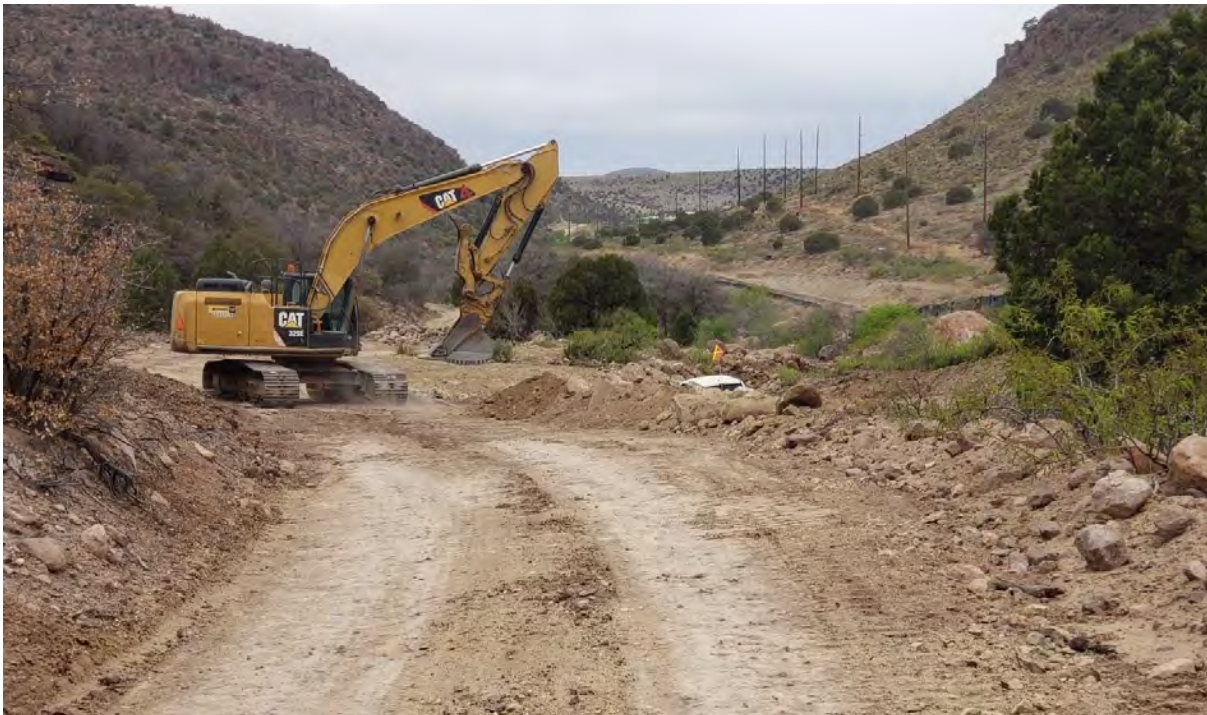
Photo 2: Crew used excavator above Lucky Bill confluence to backfill along access road.
