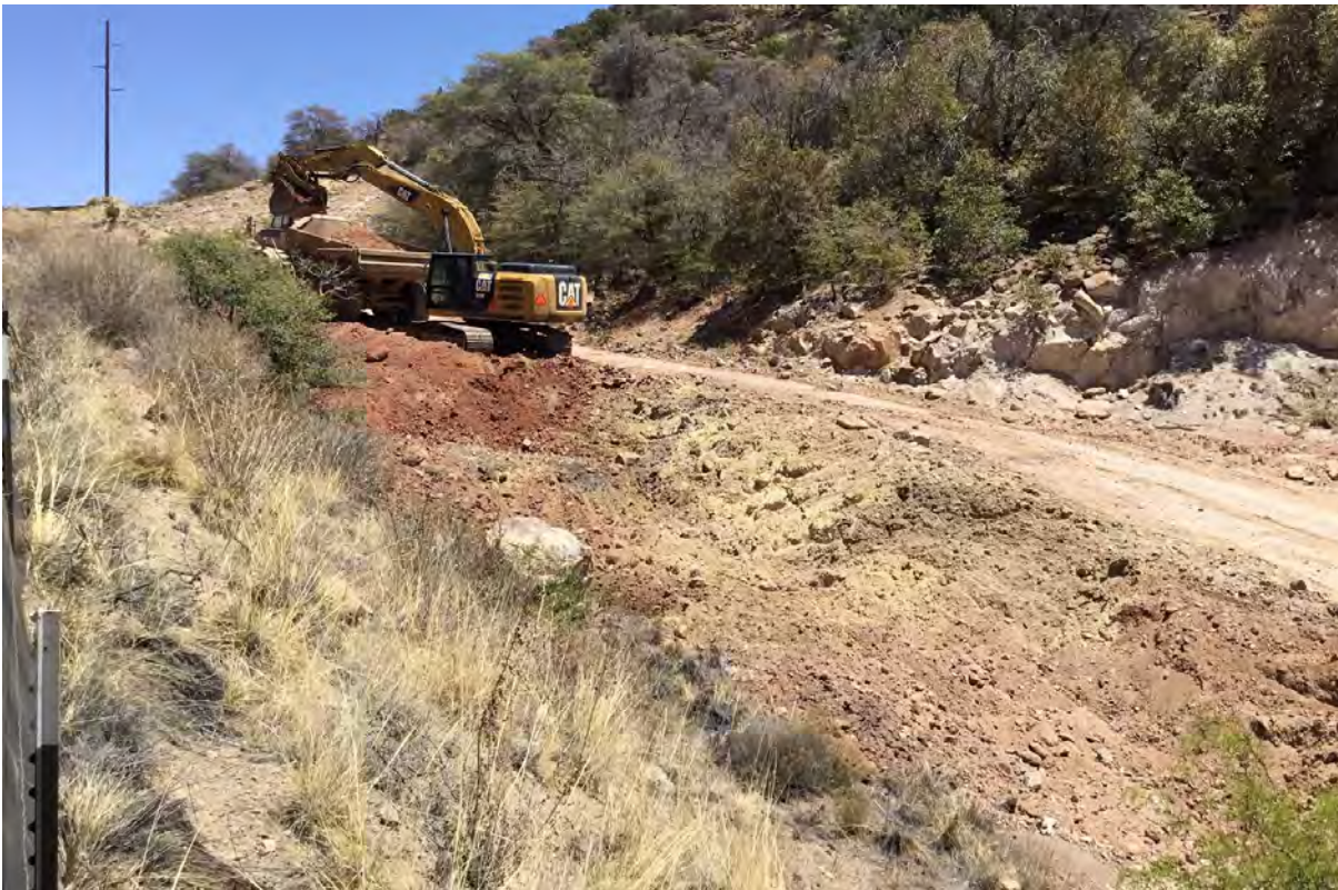
Photo 2: Crew removed red material near Shaft 1. Yellow material will be removed also.
