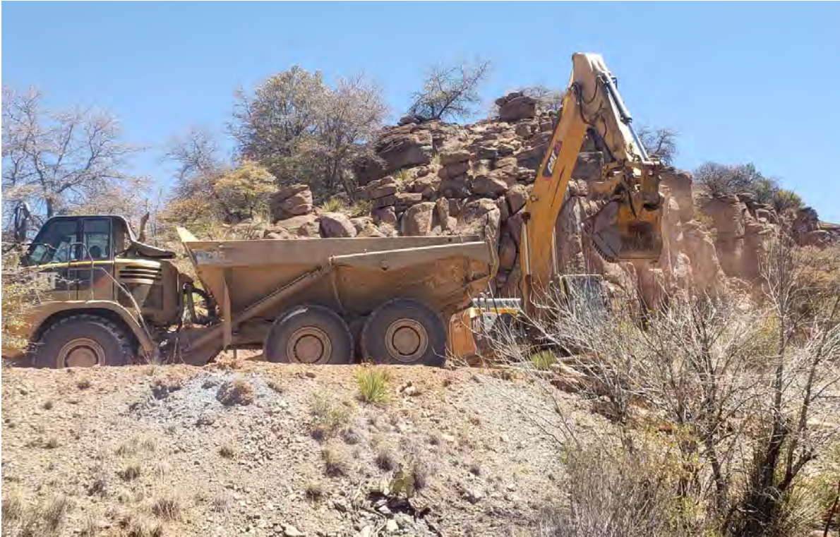
Photo 1: Shared Services continued removing material from the road near Shaft 3 at the confluence with Lucky Bill Canyon.
