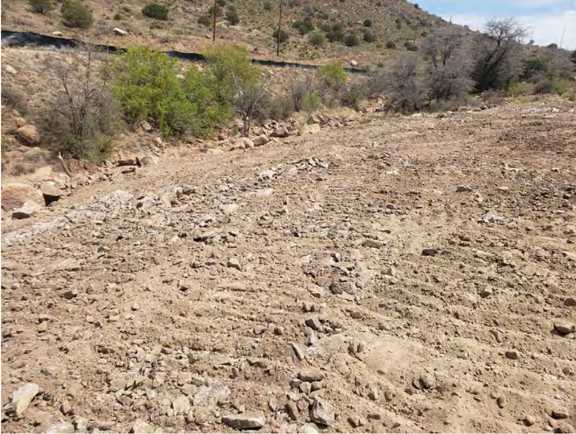
Photo 3: A well-graded slope was achieved using cover material on the creek bank that was excavated during removal. Large boulders at the toe (left) serve as armoring.
