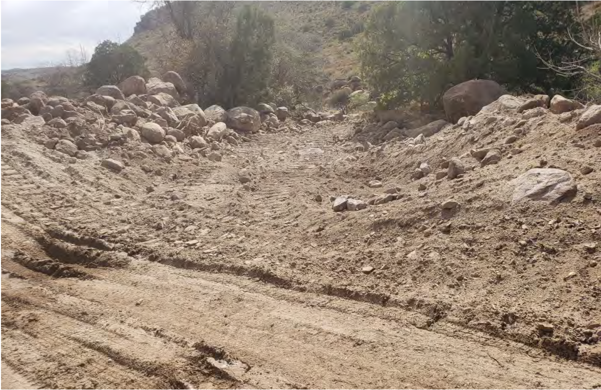
Photo 3: Boulders and sediment were removed from channel from Lucky Bill to Bayard Canyon creek
