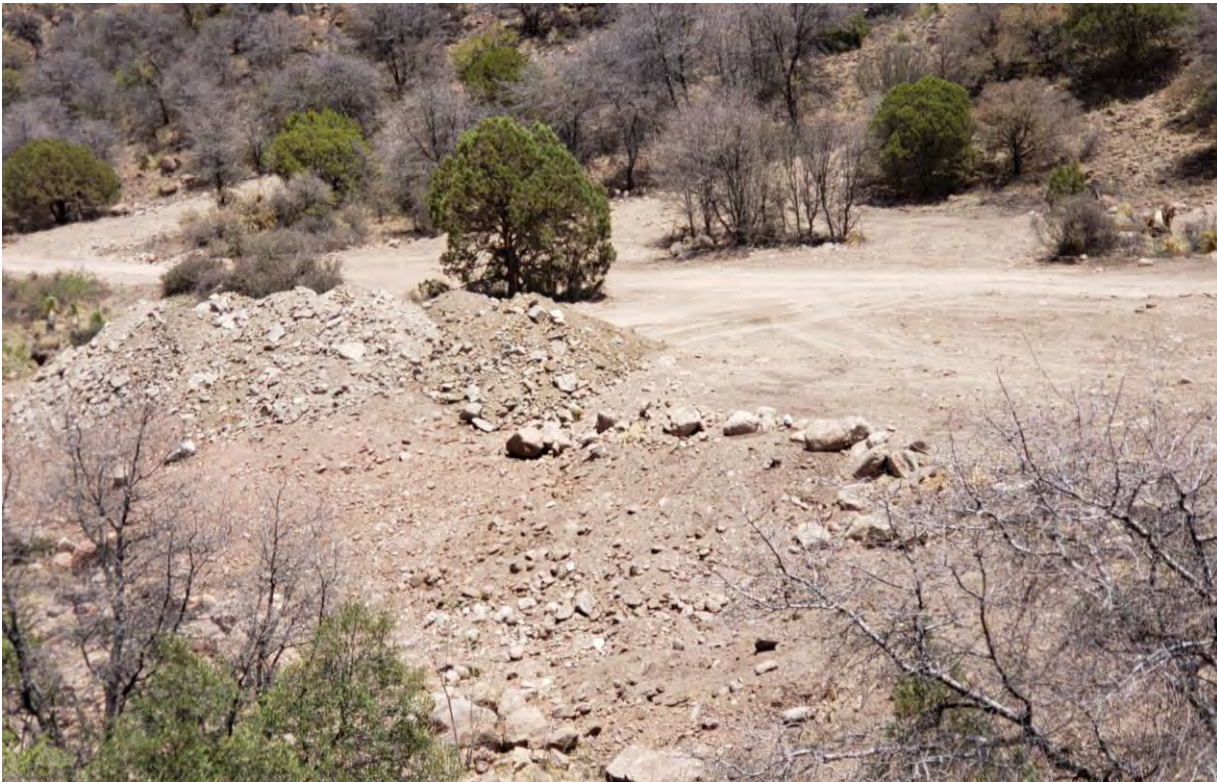
Photo 2: Crew mounded rocky cover material from Groundhog borrow area at creek bank.
