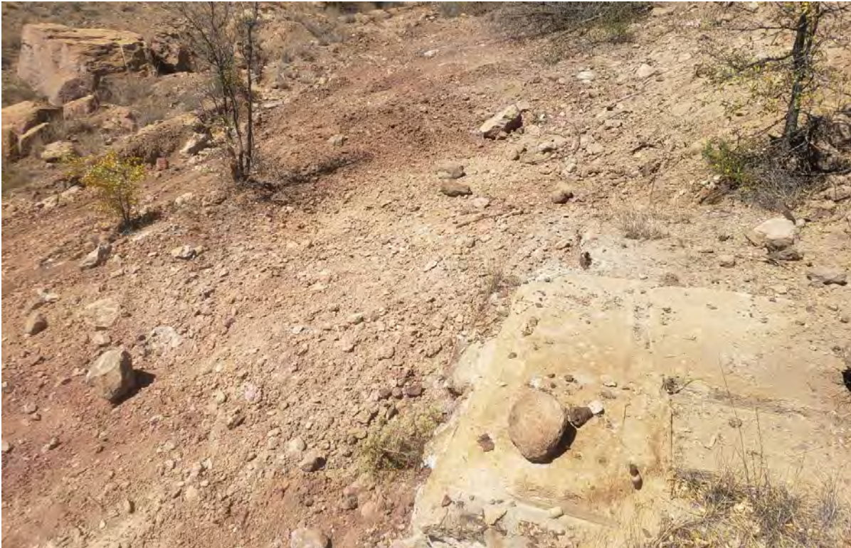
Photo 2: Crew removed red material near Shaft 2. Could not remove concrete without breaking it.
