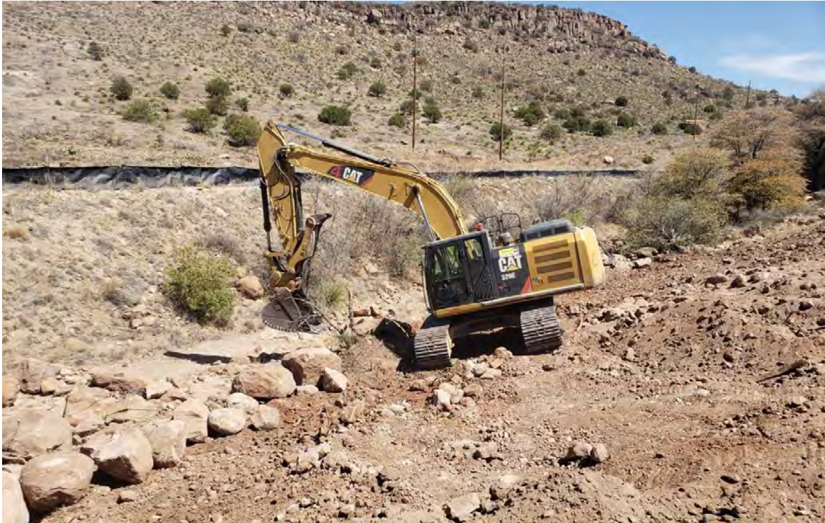
Photo 2: Primary focus of day was removing red material from creek bank west of Shaft 8 and placing existing boulders along toe of new slope for backfill stabilization.
