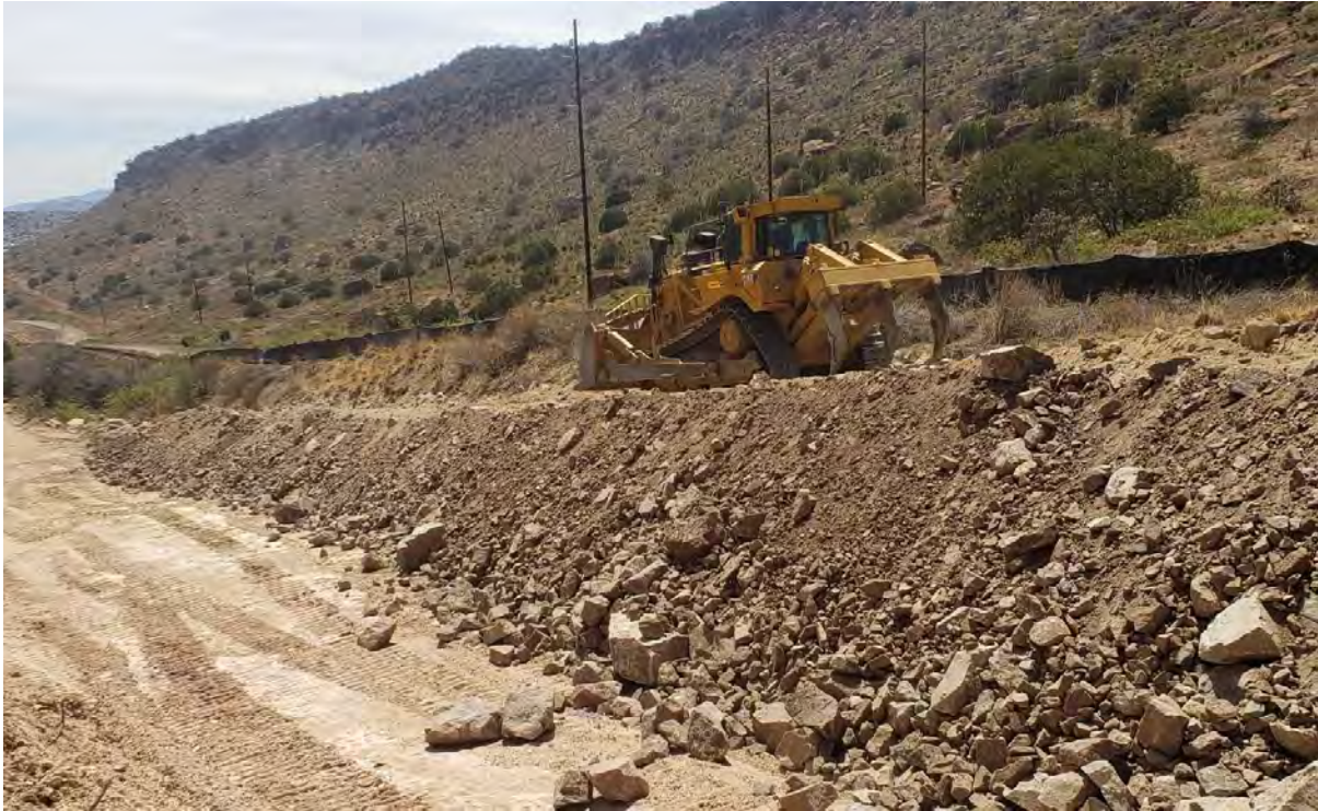
Photo 1: Shared Services continued working on ramp at north end of work area. Dozer spread layer of fine material on top of rocky material that makes up most of ramp.
