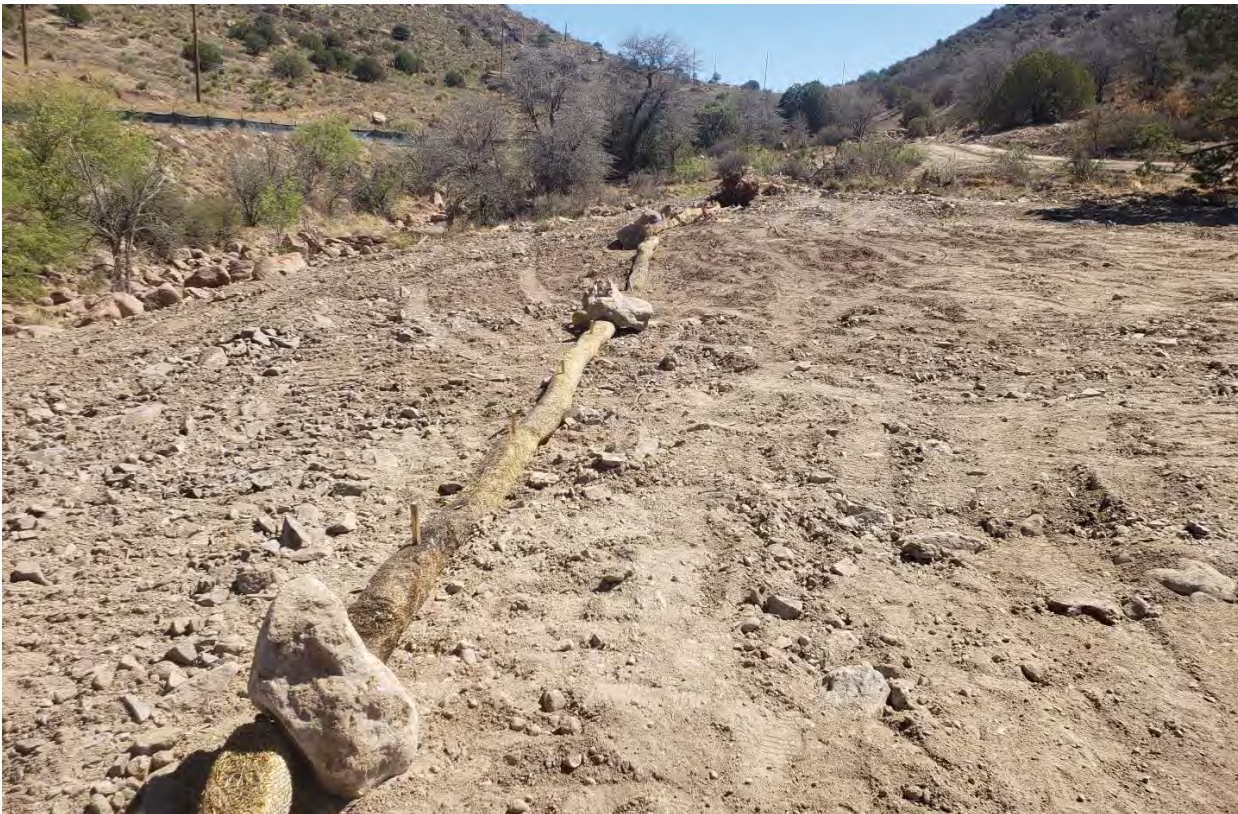
Photo 2: Straw wattles installed along creek bank – boulders and stakes used to secure.
