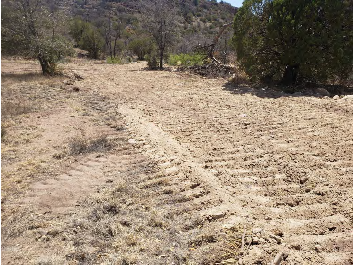
Photo 3: Backfill and final grading was completed quickly at the south end of the site.
