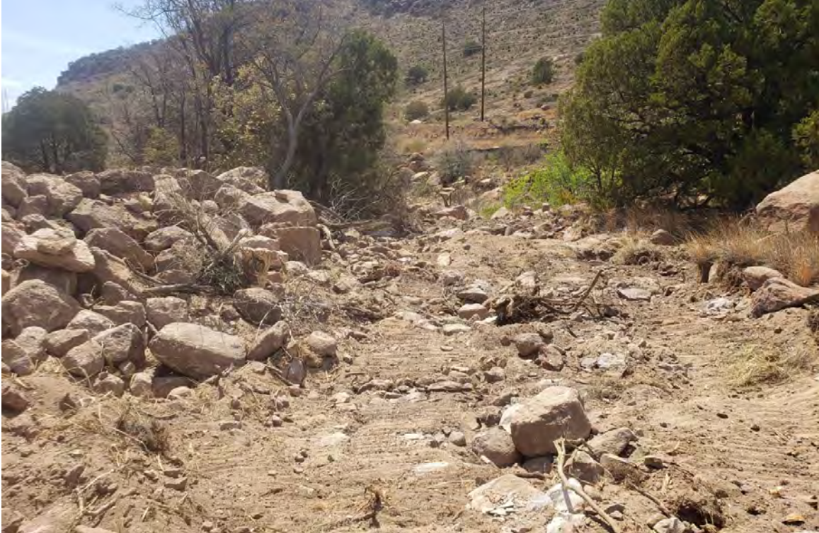
Photo 3: Crew re-established original creek channel from Lucky Bill into Bayard – using boulders (left – above) to reinforce bank.
