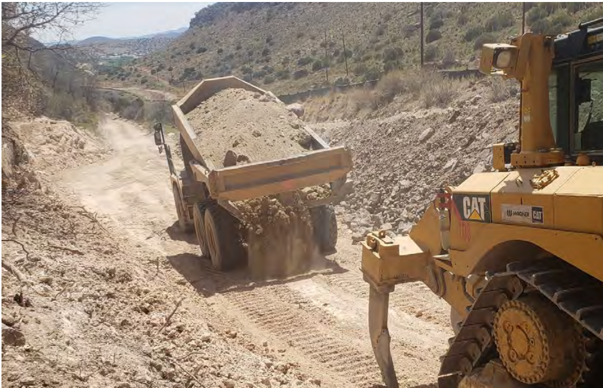
Photo 2: Crew imported cover material for placement on east bank (left) at north end of site.
