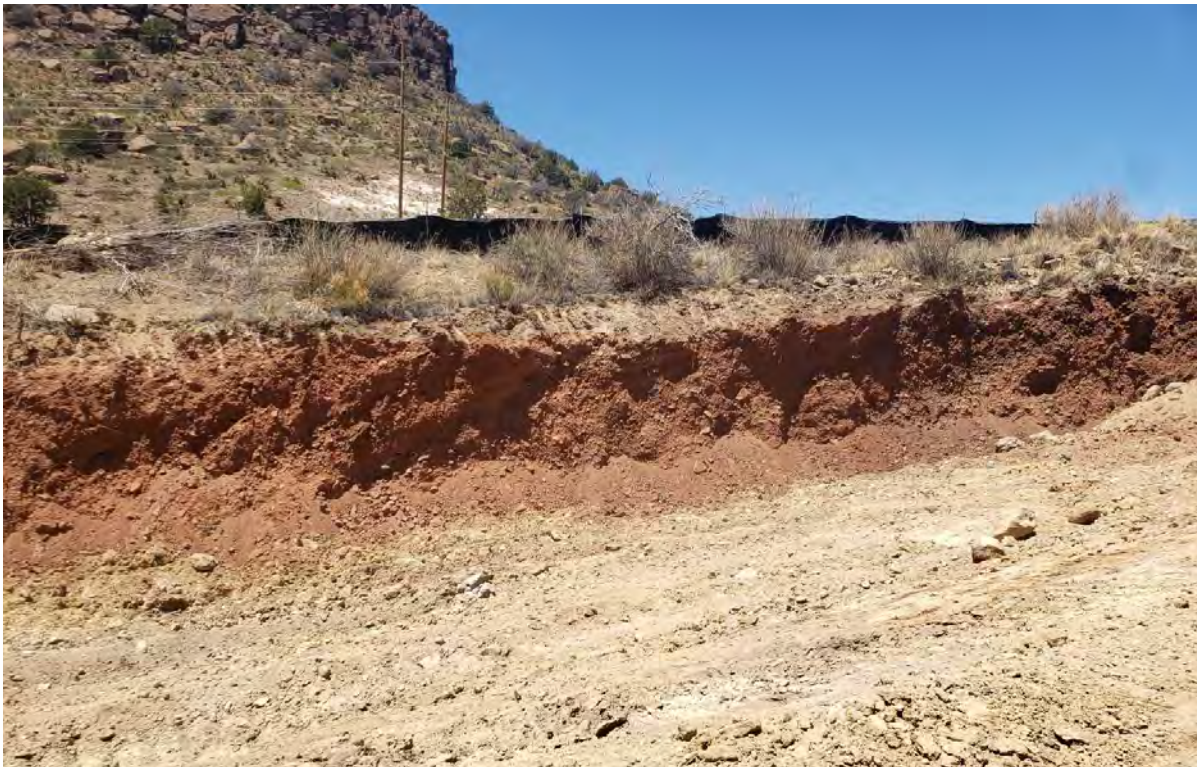
Photo 2: Crew did not remove red material along pipeline corridor near Shaft 1 out of concern for undermining. Checking with Elmo Gomez to determine how much further excavation can safely go.
