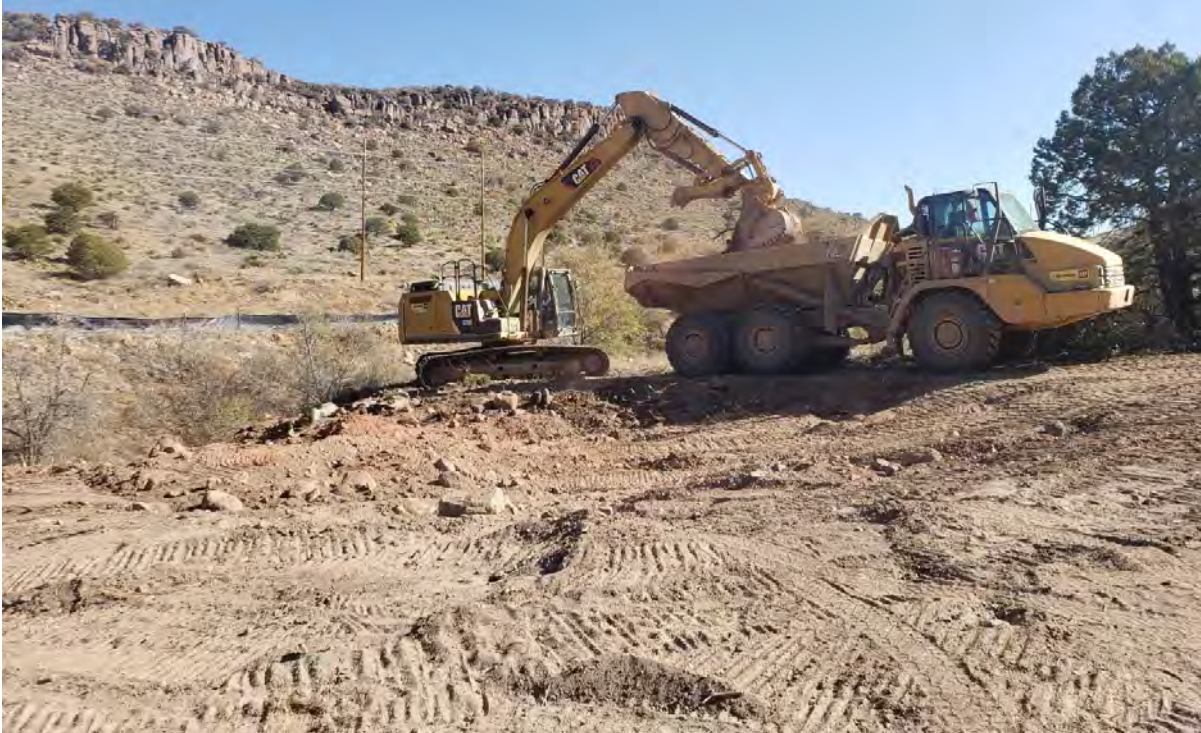
Photo 1: Shared Services continued removing red material from creek bank west of Shaft 8.
